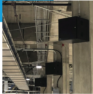
Pillar 3 Mitigate Risk with Adaptable Equipment & Cabling
