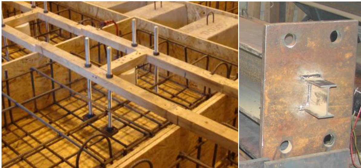
Figure 1: On the left: formwork, reinforcement, anchors and strain gauges ready for casting; on the right: column, base plate and shear lug
