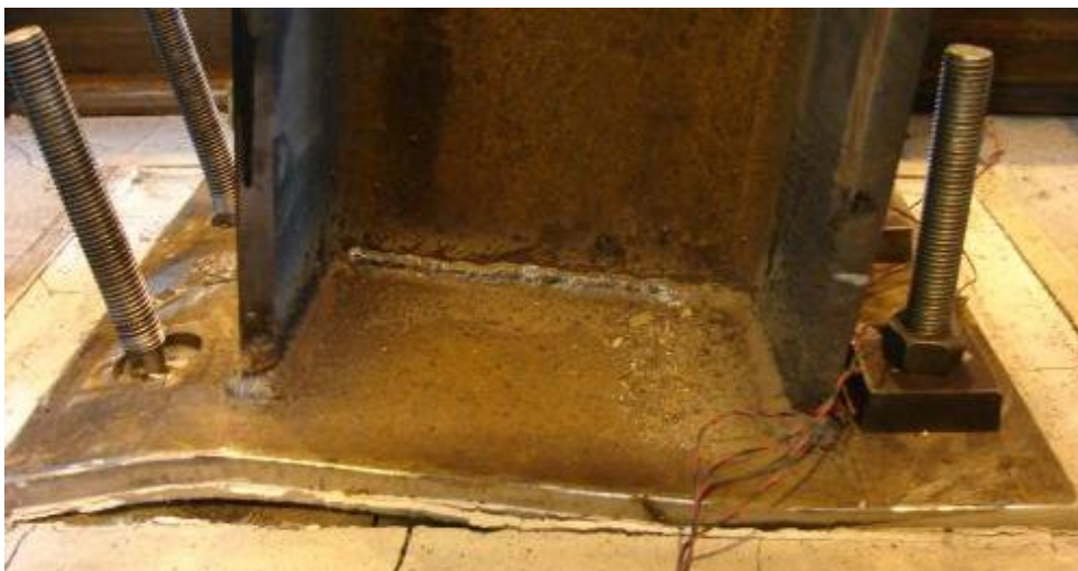
Figure 9: Joint 2 — deformed base plate and bolts after the experiment
